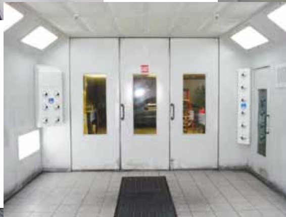
Downdraft booth with corner tower and vertical retrofit tower
