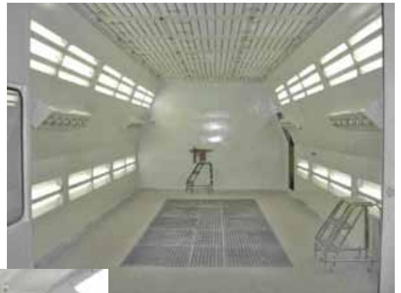
Downdraft booth with four horizontal retrofit towers
